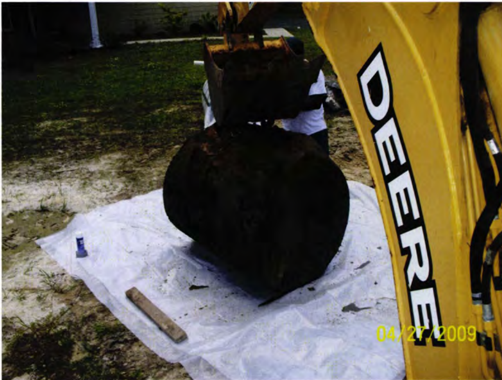
Picture 1: UST 295Birch-2 immediately after removal. UST 295Birch-1 was identical.
